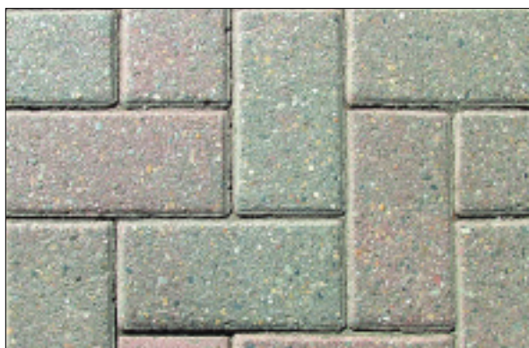
▲ Non-Durafaced Pavers showing wear and aggregate...
