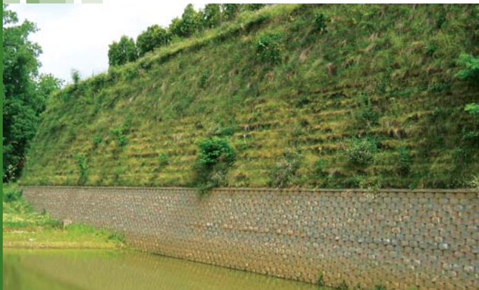
A structural and aesthetic solution is achieved at Brookworth Plaza by combining both the Mesa and SierraScape Systems.
