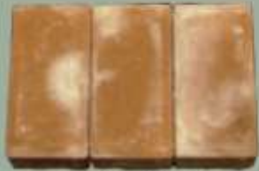
PAVERS WITH EFFLORESCENCE
