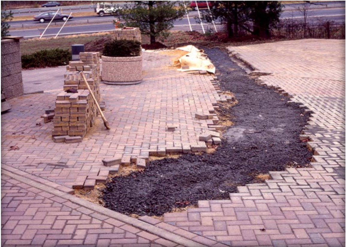
Figure 11. Trench filled with compacted aggregate base. Temporary edge restraints should be used around the opening perimeter.
