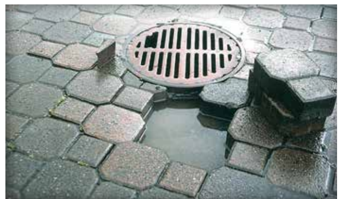
Figure 15. An absence of holes in the sides of this roof drain led to ponding.
