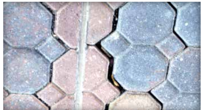
Figure 12. An absence of edge restraints and use of a sealant in this construction joint caused the pavers to shift and open their joints on both sides of the sealant.
